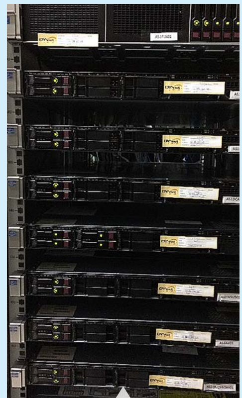
42U Rack in Data Centre – Asia (Inside)
