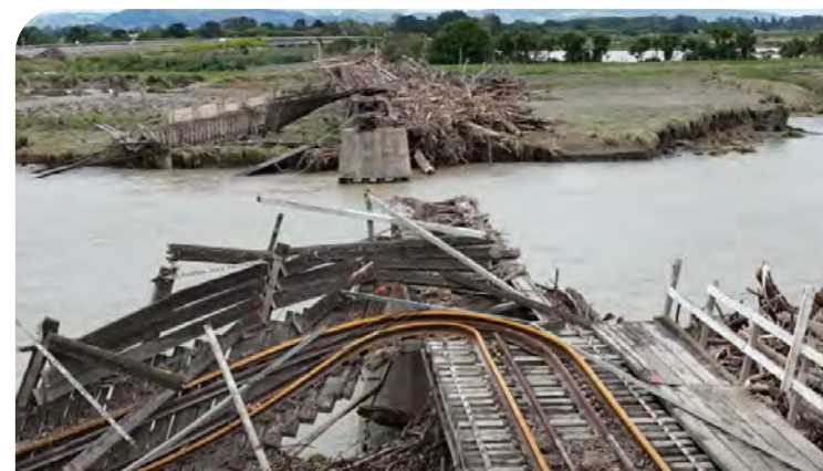
Bridge washout caused by Cyclone Gabrielle
